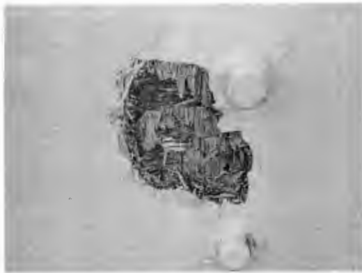
Rot on Exterior Wall Room L
