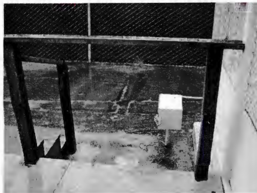
Broken Railing Room L
