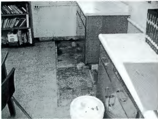
Water Damage Room K
