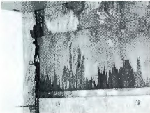
Water Damage Room K
