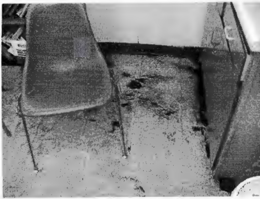
Debris from Leak Room K
