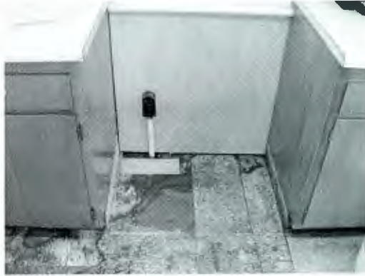
Water Damage Room K
