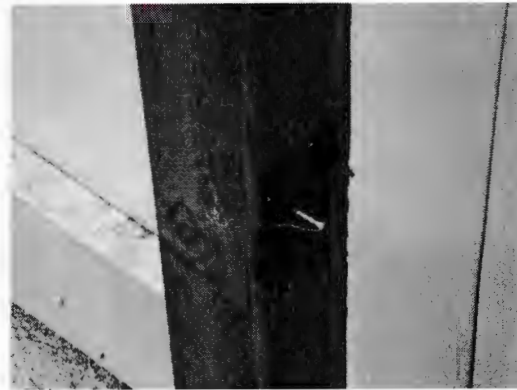
Exposed Nails Room L
