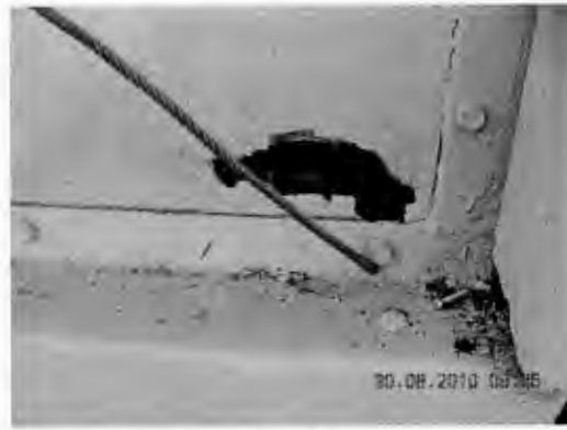
Rot on Exterior Wall Room L
