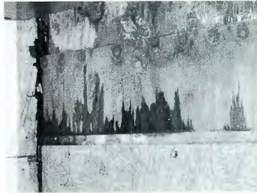
Water Damage Room K
